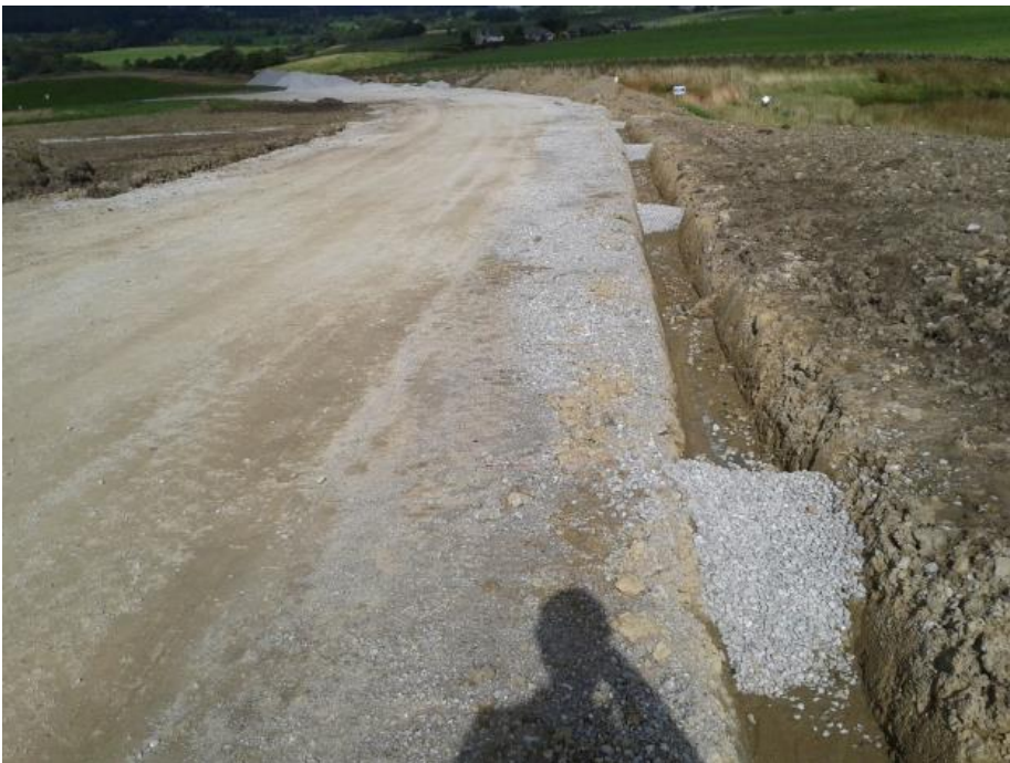
Plate 4: Typical check dams – to be installed in drainage ditches adjacent to roads
