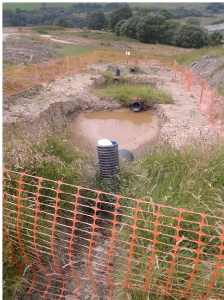
Plate 5: Typical lagoon and flocculent station
